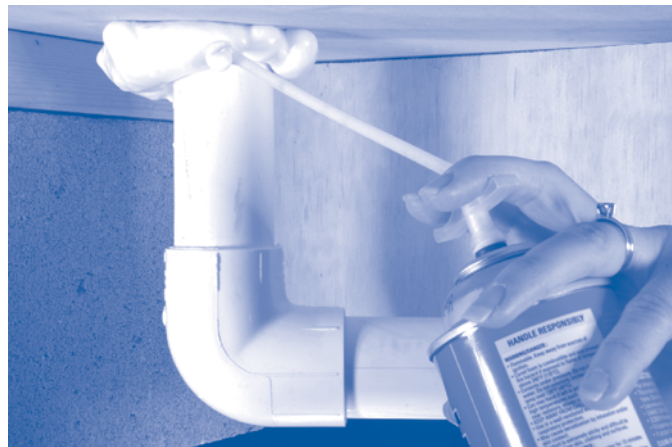
Many homes lack adequate insulation or have gaps that need air sealing.
